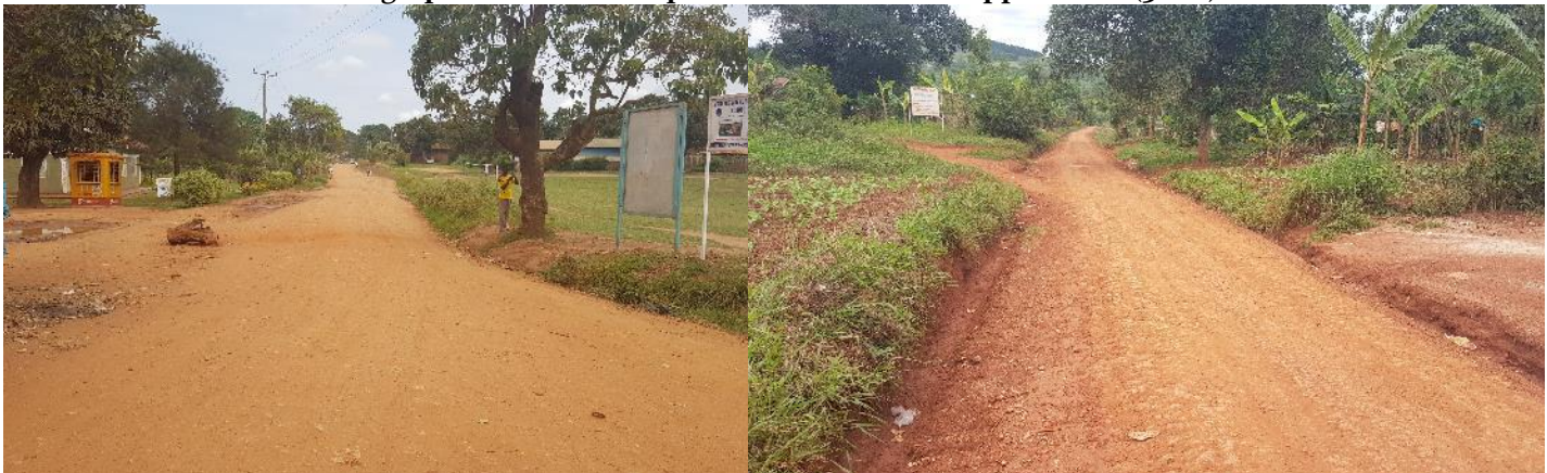
Ch. 0+000: Start of the link requiring drainage improvement Ch. 2+100: Narrow carriageway
