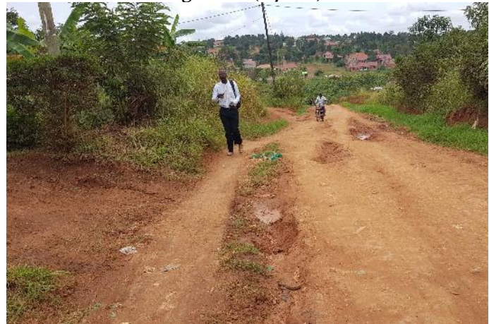
Ch. 1+000: Poor drainage
