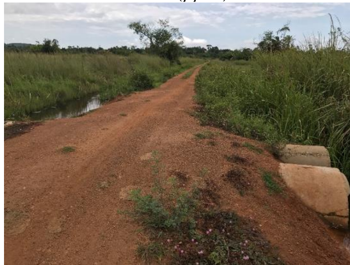
Ch. 6+700: Culvert installations without end structures
