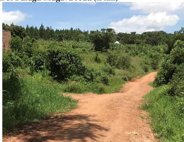
Ch. 9+500: Narrow carriageway and inadequate routine manual maintenance
