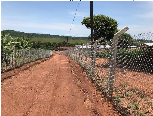
Ch. 2+100: Gulleys as a result of poor drainage
