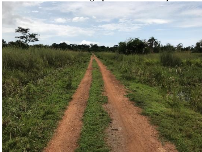
Ch. 6+200: A heavily vegetated section in a swamp as a result of lack of routine manual maintenance
