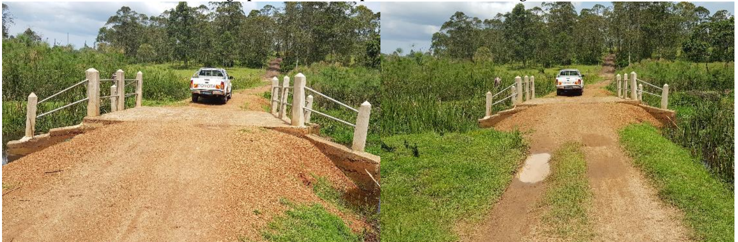
Exposed wing walls due to inadequate fill material on the Approach road River training required up and downstream
