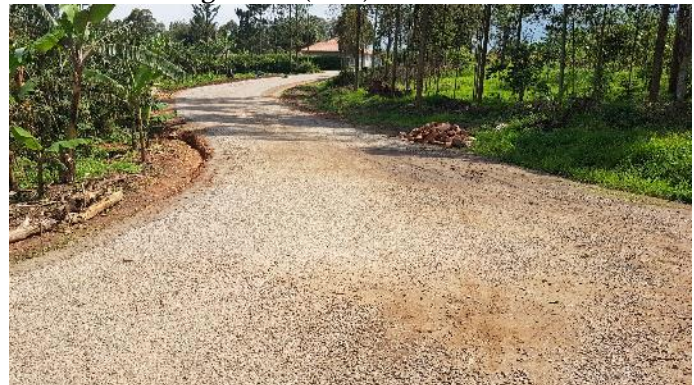
Ch. 0+600: Culvert installation urgently required
