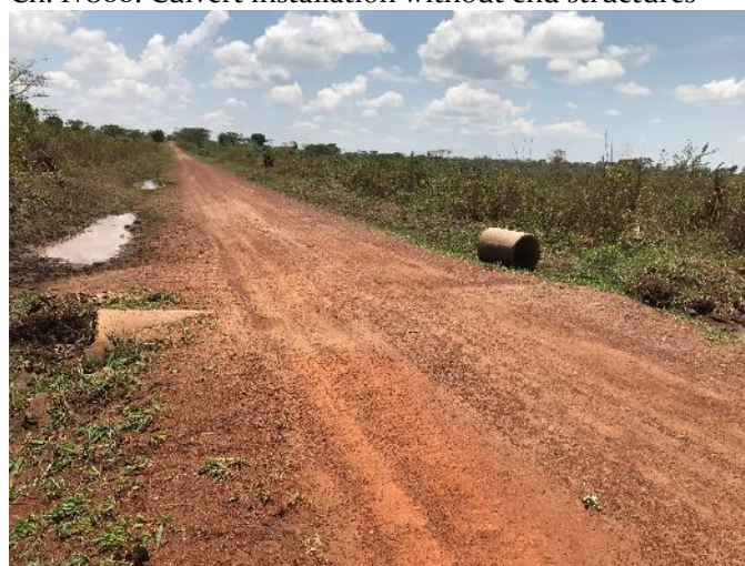
Ch. 6+200: Culvert installation without end structures, inadequate backfill and idle culvert pieces
