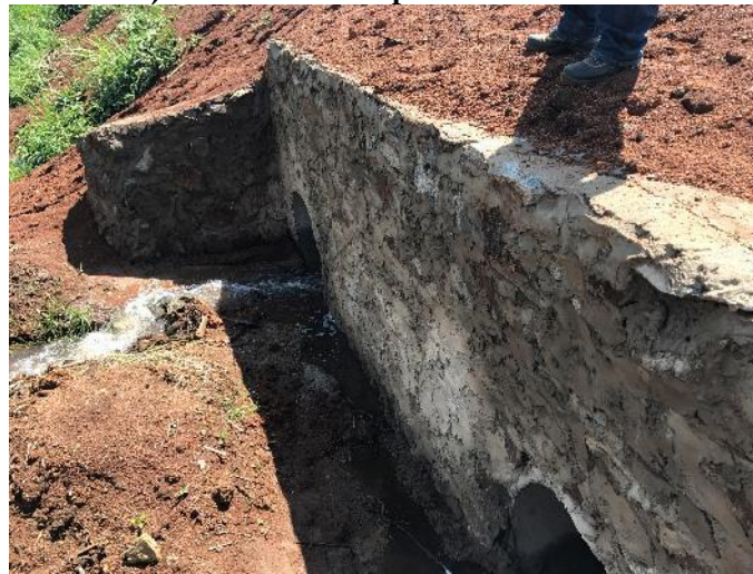
Poorly constructed splash aprons
