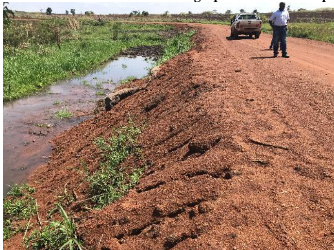
Loose gravel embankment as a result of lack of compaction
