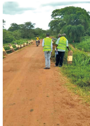
UNRA Moyo: Narrow and aged bridge with damaged guardrails on Moyo – Obongi road – Guardrails to be replaced for safety of road users. Plans are underway to design and construct a new bridge.
